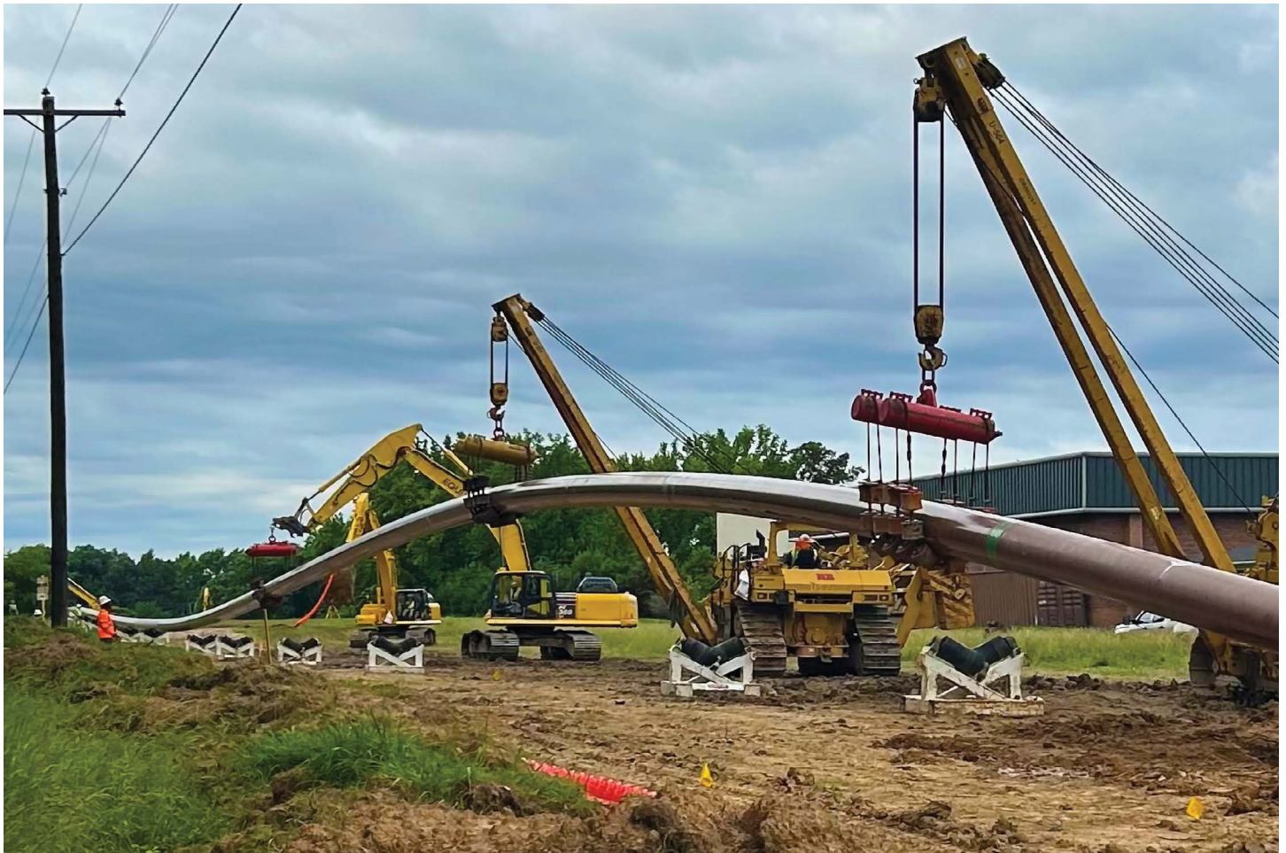
The Weaver-Gill Pipeline was a 5.4-mile, $30 million modernization project to improve the pipeline distribution of natural gas in South Memphis.
