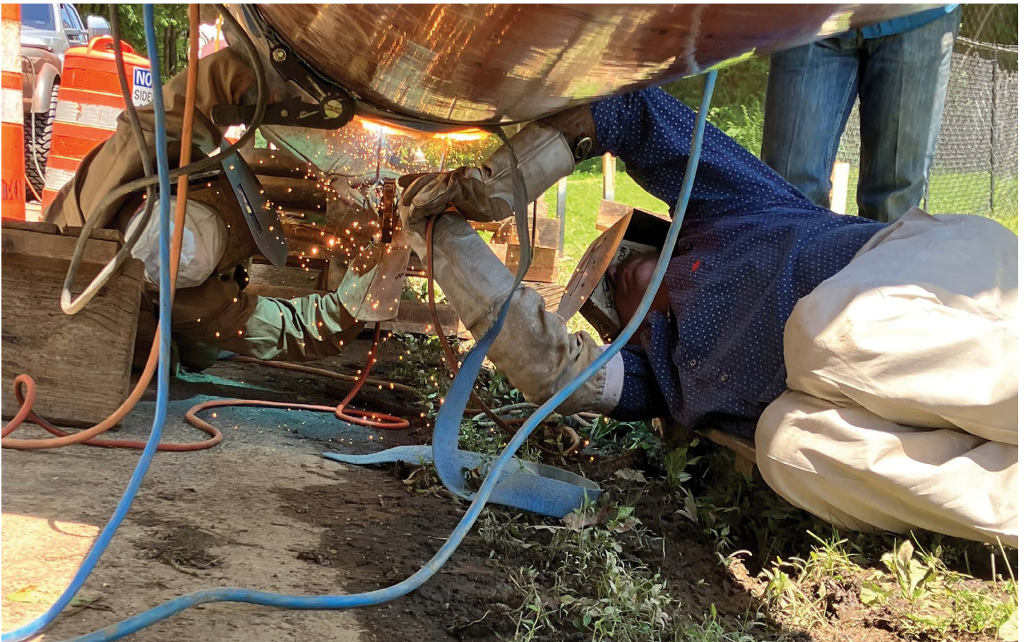
The Weaver-Gill pipeline—made of thicker, stronger steel pipe—is the last MLGW Way Forward capital project and one of the biggest modernization projects that MLGW has ever done.
