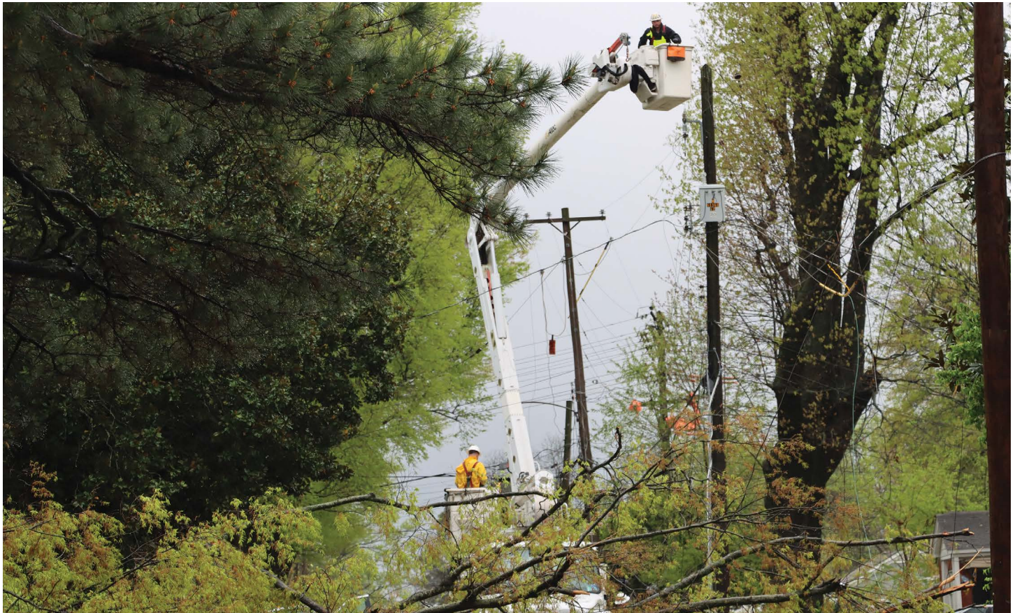
After several years of playing catch up, MLGW's tree trimming crews are now back on a three-year trimming cycle. Their efforts help reduce power outages and improve service reliability for our customers.
