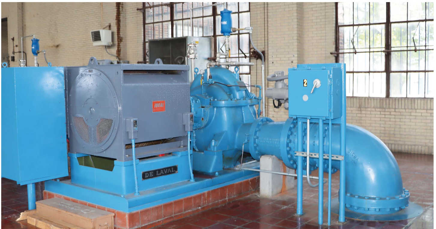
The Sheahan Pumping Station was built in the 1930s on an old plantation and consists of three separate buildings—one for pumping, one for aeration and another for filtering.
