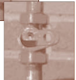
Closed Gas Meter
