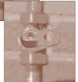
Closed Gas Meter
