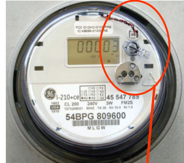
Smart meter (Smart Grid Demo)
