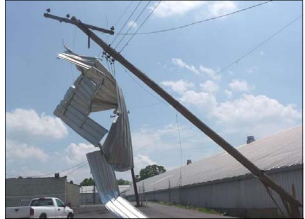
High winds tore off this sheet metal roof and snapped a utility pole in North Memphis.
