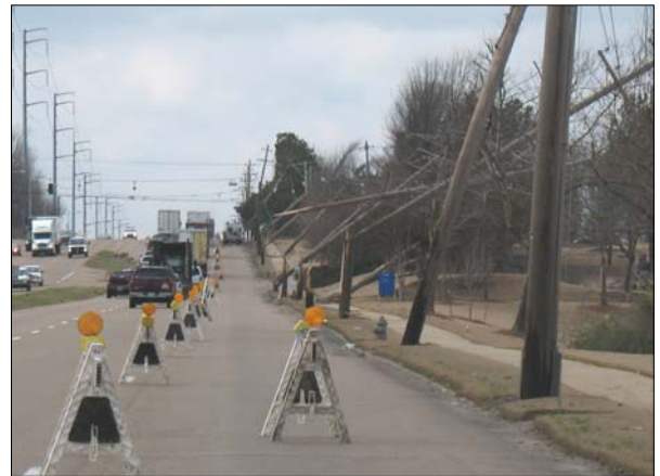
This view of Shelby Drive and Malone Road illustrated damage to utility distribution poles snapped by strong winds.
