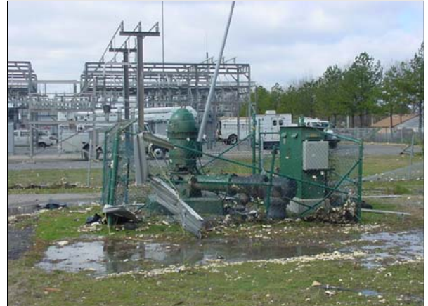
View of damage at MLGW’s substation 71 in Hickory Hill area. The substation sustained shrapnel-like damage from flying debris, as well as the loss of electric transmission lines feeding into the facility.
