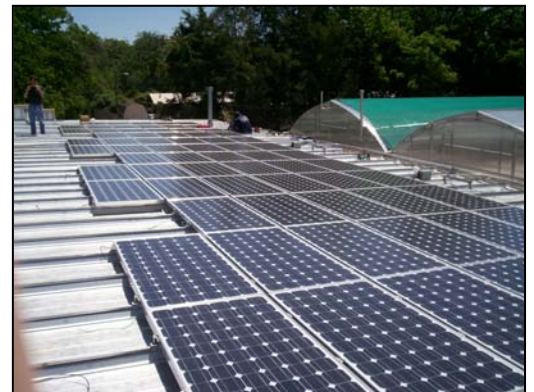
Example of a flat, roof-mounted 10 kW-capacity solar array
