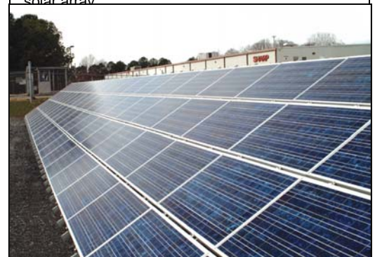
Example of a 50 kW-capacity solar array installed at ground level on angled mounts, facing south
