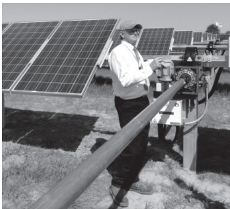
A representative from the installation company, Lightwave Solar, discusses the new Solar Farm system.
