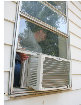
MLGW employee David Pace (inside window) helps a customer battle the heat by installing a window air conditioner.
