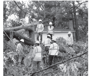
MLGW crew cuts away at storm damage.
